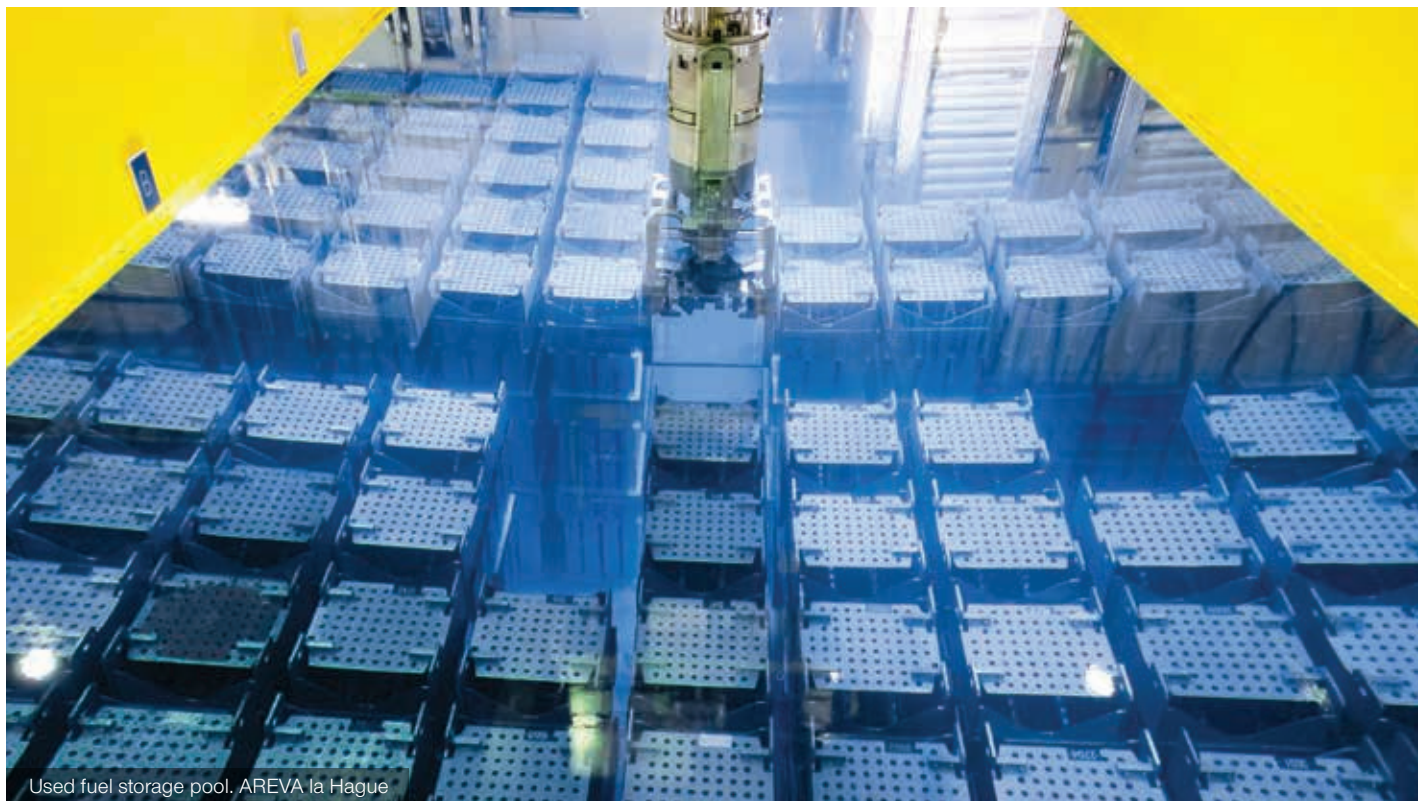
Used fuel storage pool. AREVA la Hague
