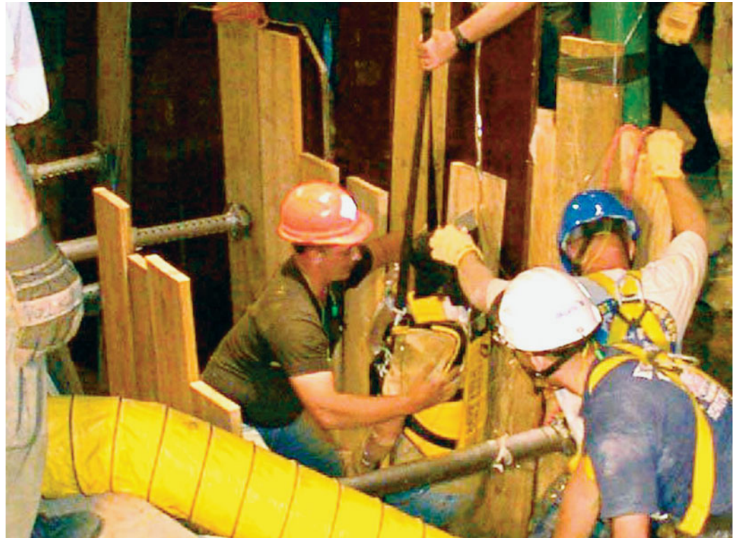
FIGURE 11-10 Patient entrapped in trench cave-in being lifted out along the long axis of the body. (Courtesy of Roy Alson, MD)
